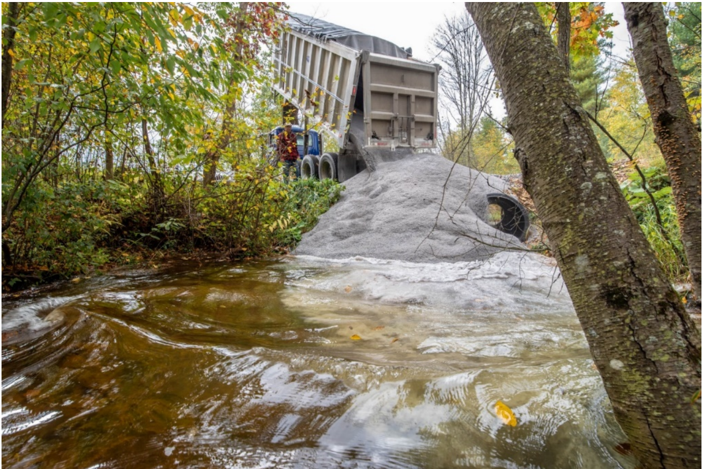
Figure 5. The last load arrived on October 12. It was the inaugural first load directly placed into the West Branch of Jones culvert pool. Photo by Brett Whitling, Clarion News.
